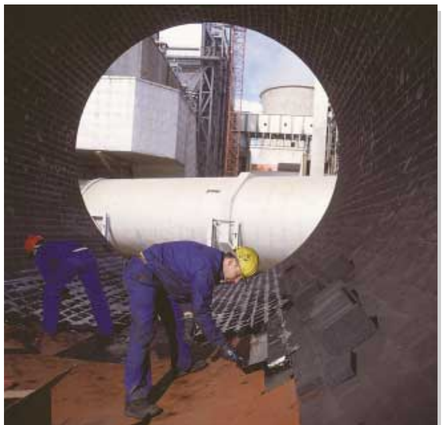
The ducts have a diameter of 6,2 metres.
