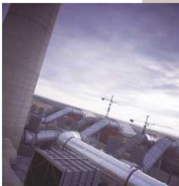
The FGD inlet and outlet ducts.
