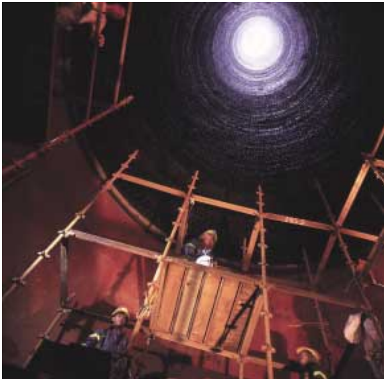
One of the steel flues after the installation of the Pennguard® lining.
