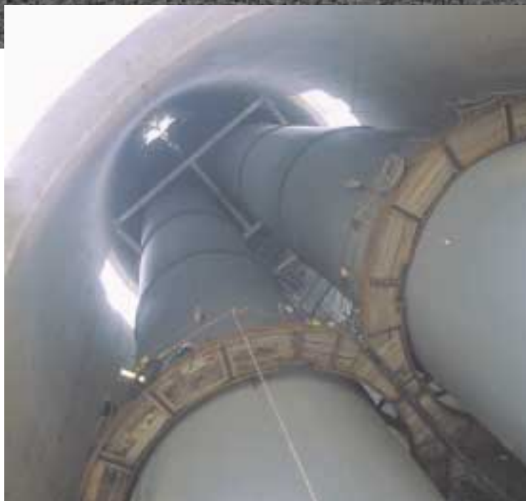
The two steel flues, each 176 m long
