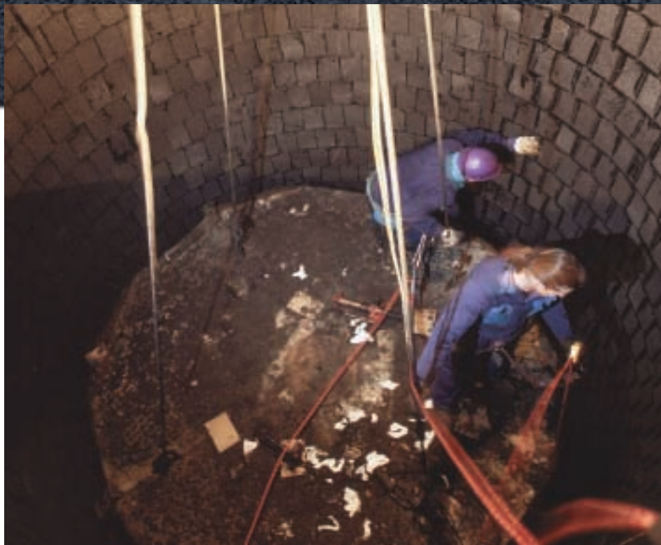
A high quality application was achieved in spite of time pressure and challenging conditions.
