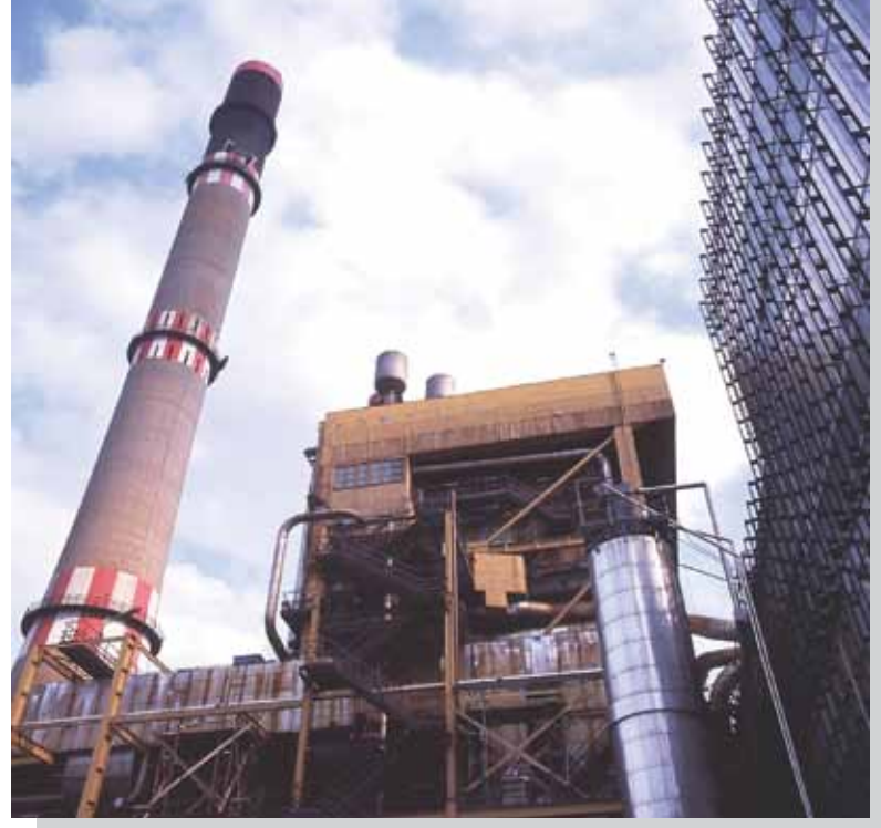
One of the 200 MW oil fired units.
