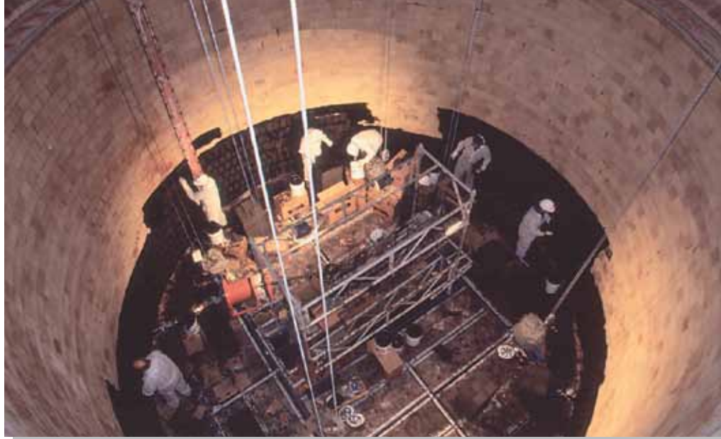
All work in the chimney was done from a movable work platform.
