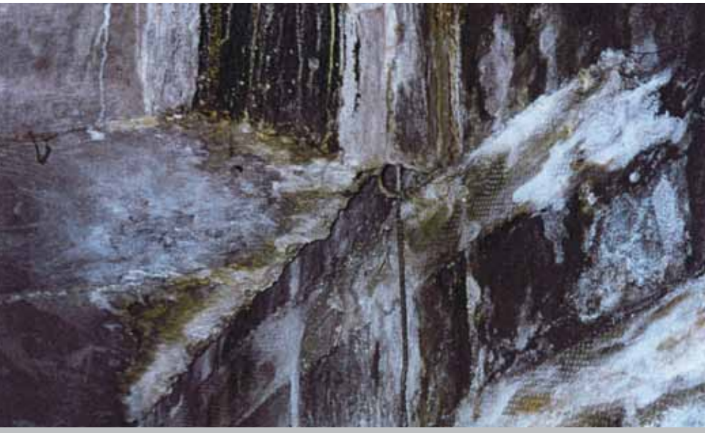
Acidic deposits on the outside of the brick flue.
