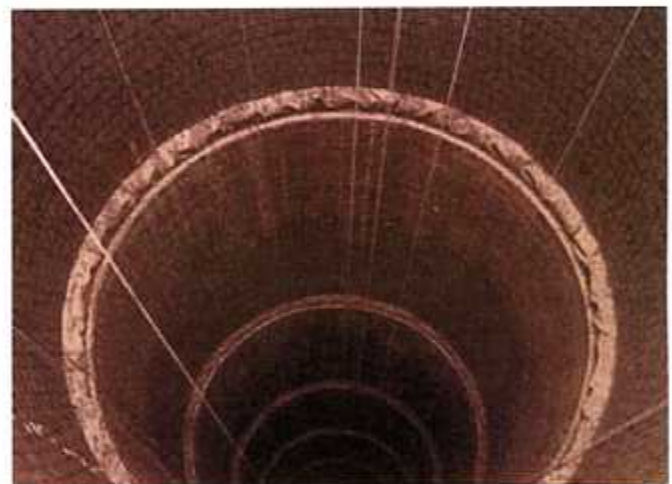
Figure 14 – Pennguard® lined flue
