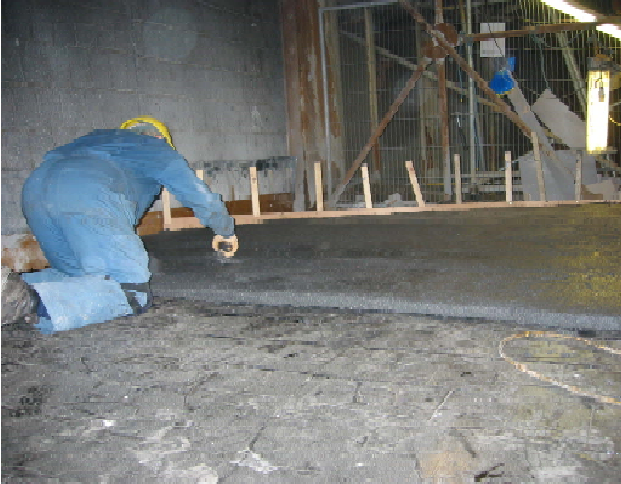
Figure 16—At the bottom of the flue, a protective layer of Tufchem ® cement is applied over the Pennguard ® Blocks
